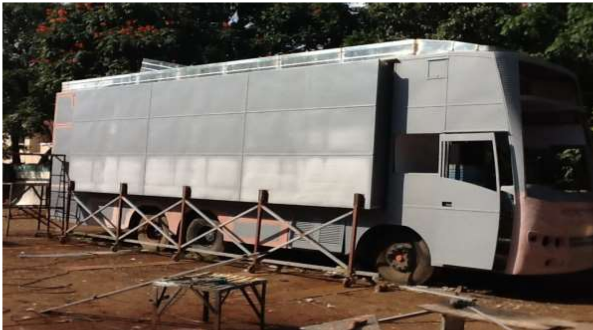
Figure 2a Five landing wheels which were assembled/attached to the outside body of expandable portion before the expansion is moving outward during expansion
